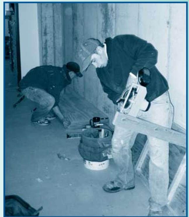
Cutmore Construction carpenters John Hinman (foreground) and Jeremy Hine (rear) work on shelving installation in the new storage space.
